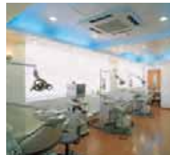
4-way Ceiling Cassette Type
